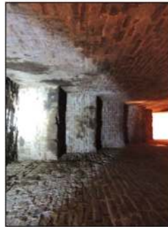
Figure 7: Masonry section infested with bats
