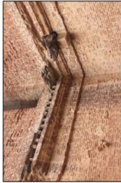
Figure 5: Deteriorated upper floor.
