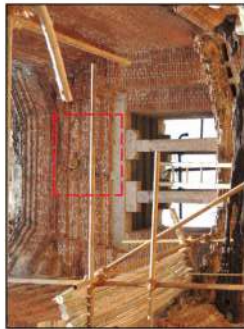
Figure 1: Deterioration in brick masonry, the second floor
